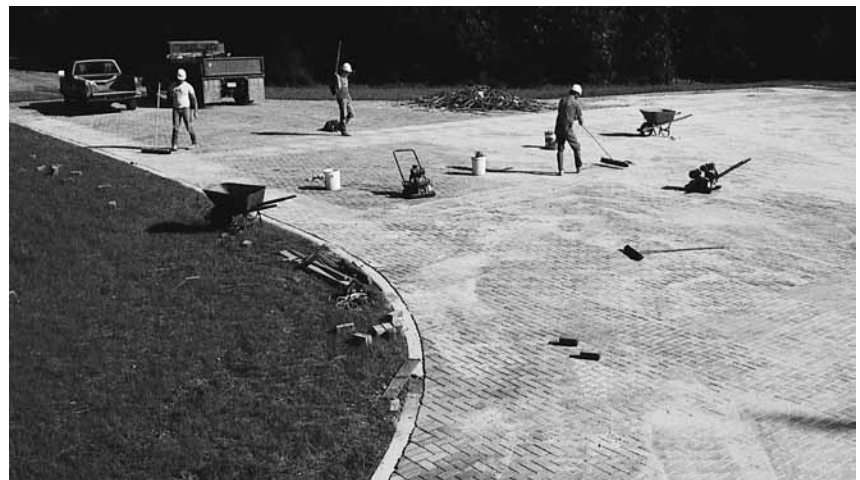
Figure 12. Excess sand swept from the finished surface will make the pavement ready for traffic.
